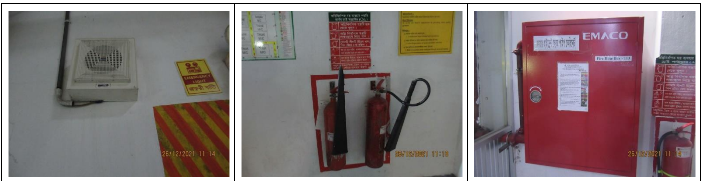
Emergency Light Fire Extinguishers Fire Hose Box
