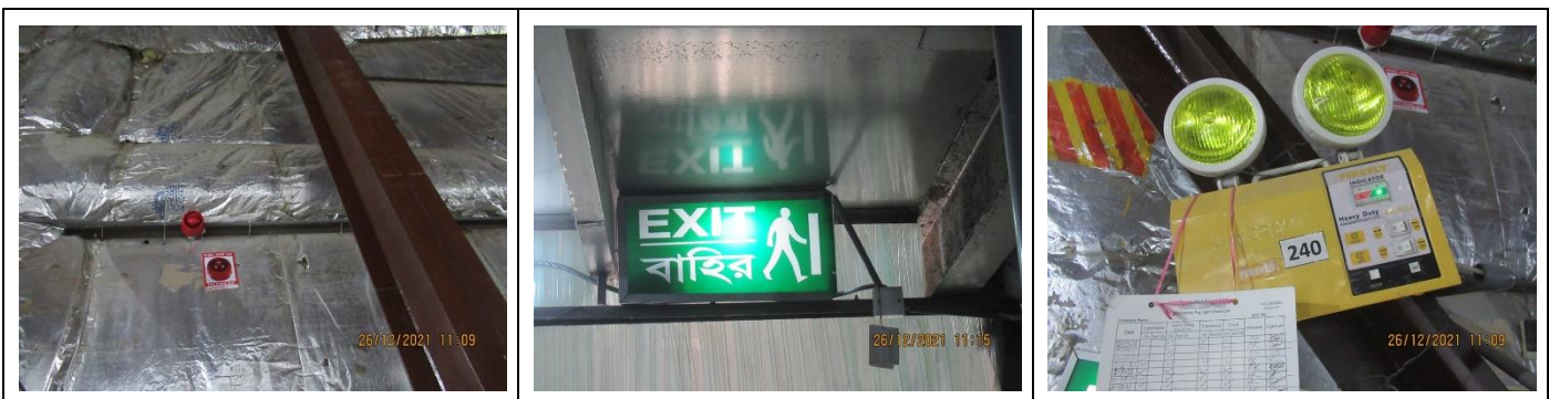
Fire Alarm Bell Exit Sign Emergency Light
